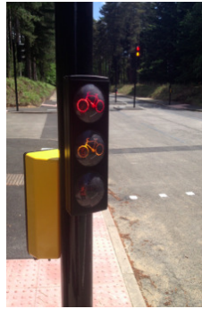
Cyclists' traffic lights
